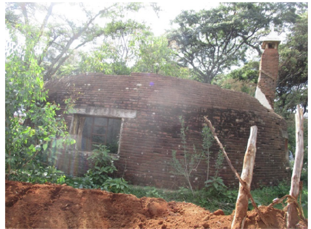
Photo 1: Destroyed storage (Former H.I.M Hailesilassie I lodge in Wolayta Sodo).
